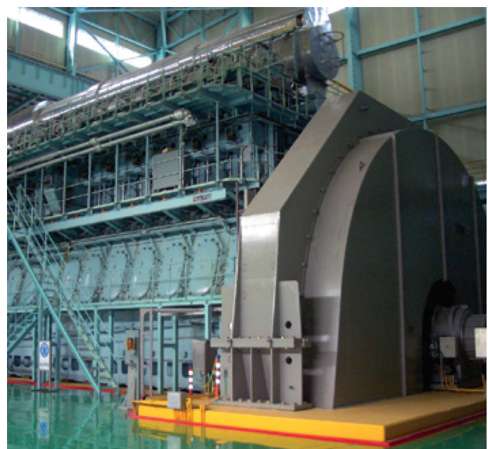
50MW stationary diesel engine at Korea Midland Power. (MAN Diesel & Turbo)
